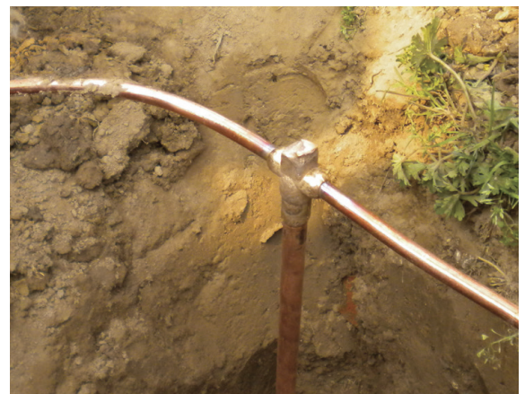
GT Cadweld connection
