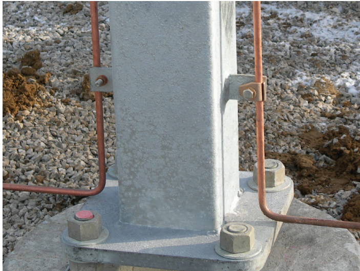
Substation earthing riser
