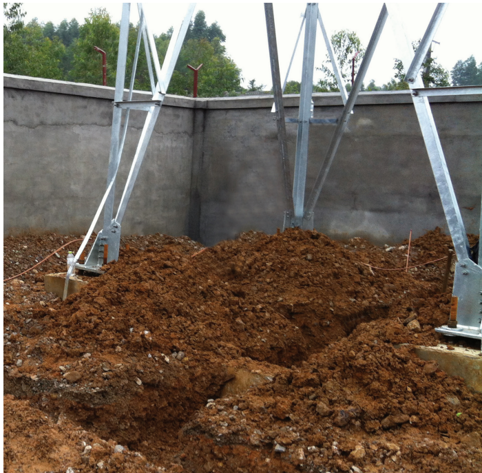
Telecom tower grounding
